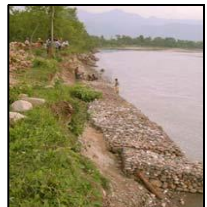
Encased stone flood defence barrier in Nepal
