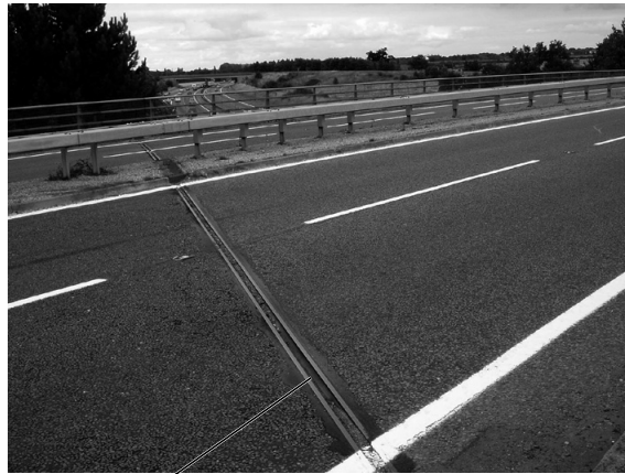
gap in bridge
