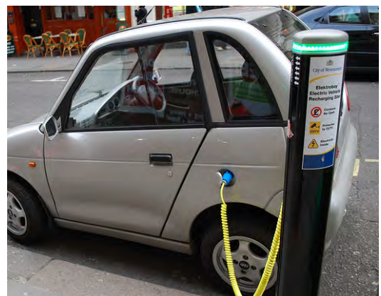
Electric car charging point
