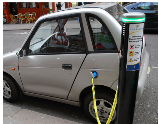
Electric car charging point
