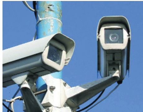
Close Circuit Television (CCTV)
