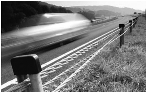
Wire rope barrier
