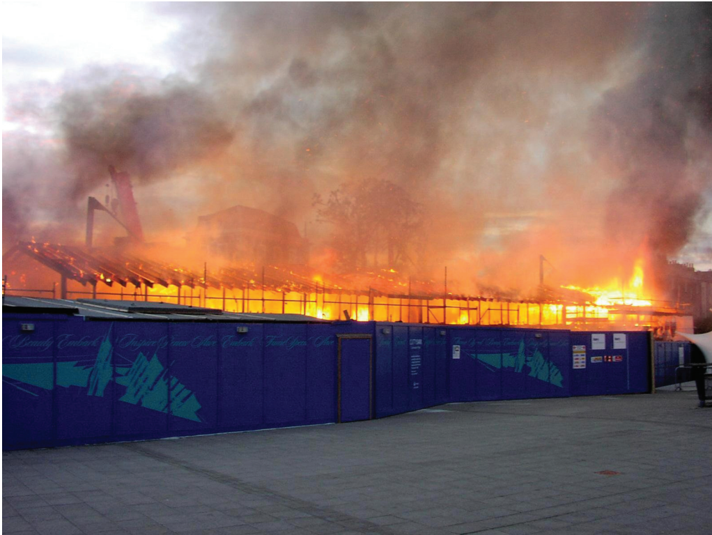
History ablaze: the Cutty Sark at the height of the fire
