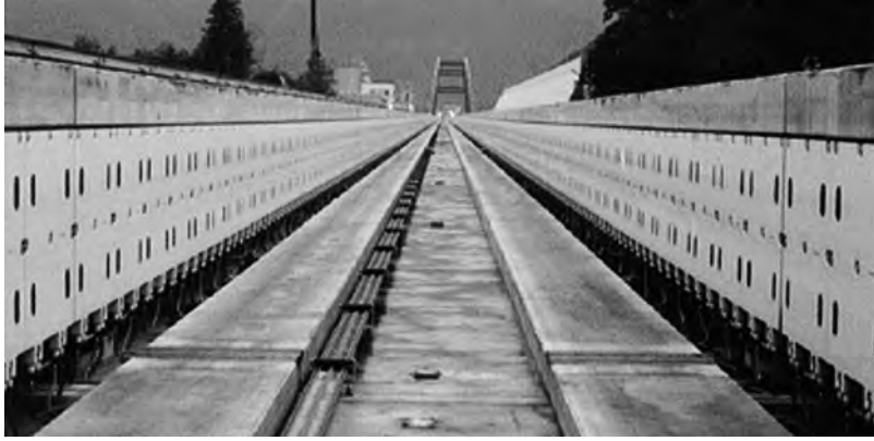
Fig. E1.2 An image of the guideway for the Yamanashi maglev test line in Japan
