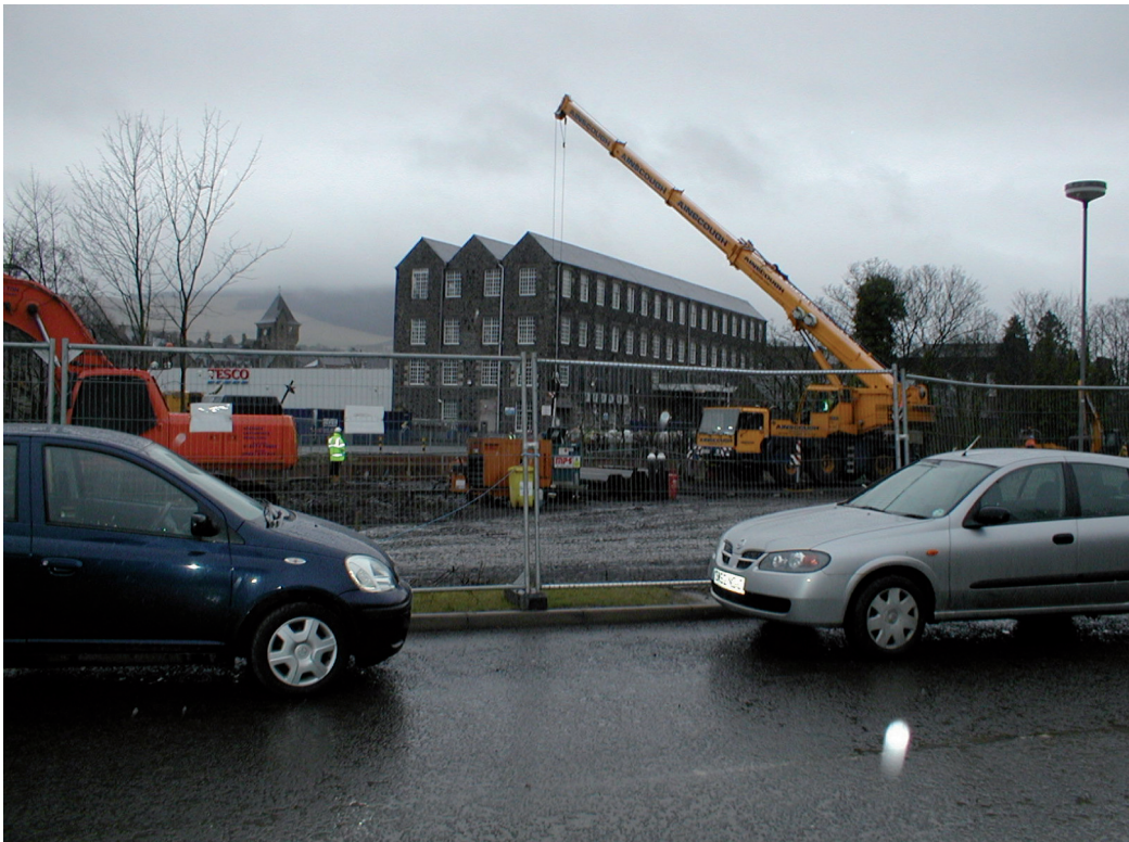
PHOTOGRAPH E Construction of a new Asda store in Galashiels, with a former textile mill in the background
