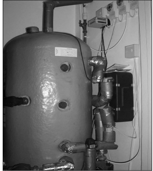
Hot water tank
