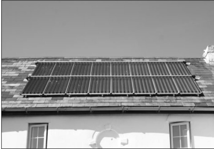
Photothermal solar panels
