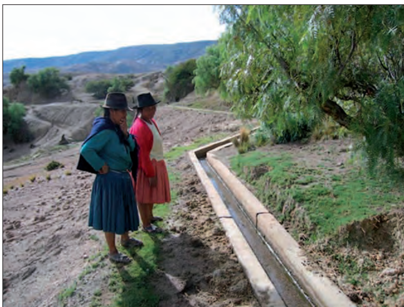
Figure 19 An irrigation channel in Bolivia
