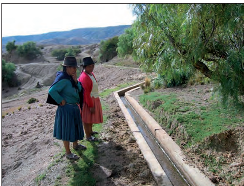
Figure 19 An irrigation channel in Bolivia
